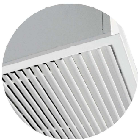
Detail of exposed inlet grille
